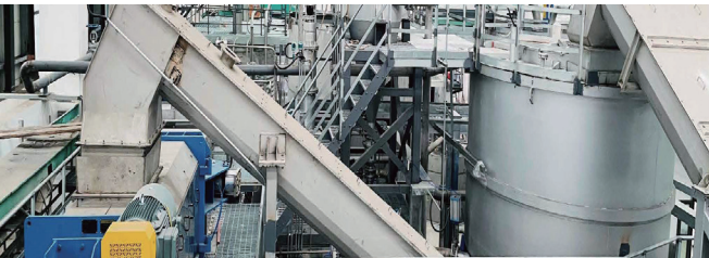
Changping Organic Matter Ecological Treatment Station Upgrading Food Waste Pretreatment Project, Beijing. Capacity 300 tons/day. (2024)
