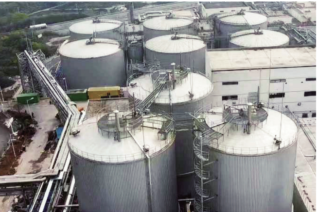
Luoqi Kitchen Waste Dry Anaerobic Project, Chongqing. Capacity 300 tons/day. (2023)
