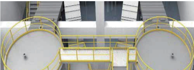
Fengtai District Circular Economy Industrial Park Food Waste Pretreatment Project, Beijing. Capacity 720 tons/day. (2024)
