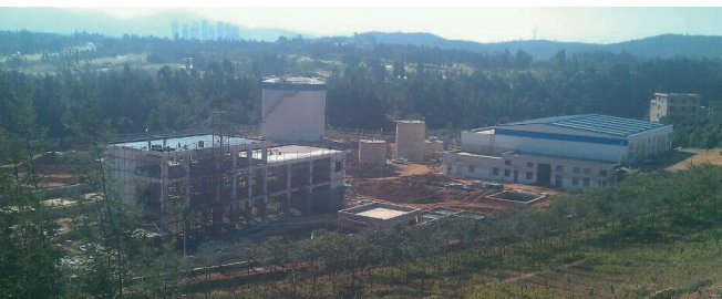
Kunming Food Waste Treatment Project. Capacity 250 tons/day. (2013)
