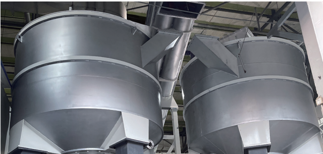
Nangong Food Waste Hydraulic Pulping Pretreatment Project, Beijing. Capacity 400 tons/day. (2022)
